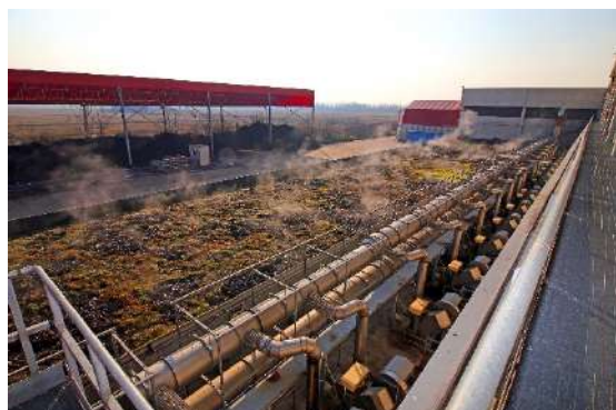
(3) BIOFILTER FOR THE ODOUR PROCESS AIR ABATEMENT
